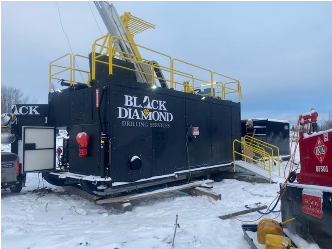
Figure 1 – Image of a Black Diamond drill rig, in operation, in northeastern Ontario, Canada
